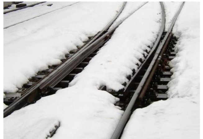
How the switch with electrical heating looks in the winter time
