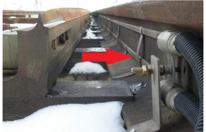
The red arrow points to the electric heating elements on the rail
