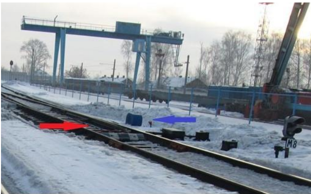
The switch at the Pozim station. The red arrow points the air pipes to the switch blade. The blue arrow points the box and the connection for the air hose.
