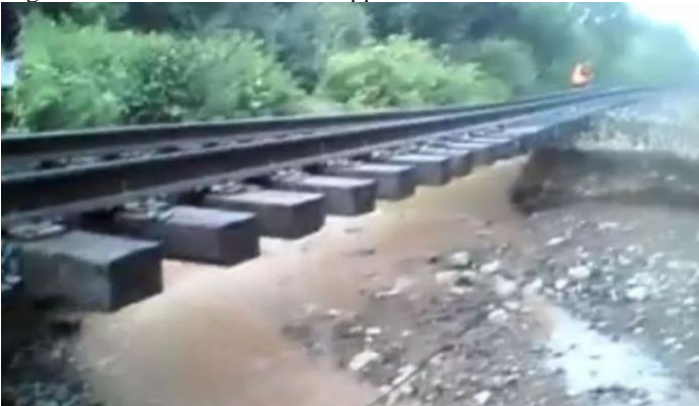
The rails and ties up in the air. It is the place where the water washed off the track.
