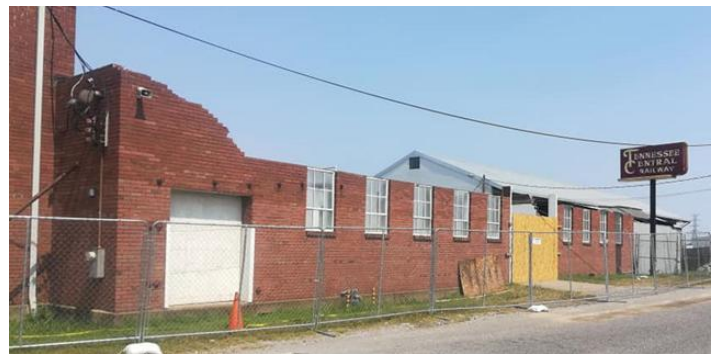
Photo by Jason Sharpe – demolition- roof trusses and bricks above windows removed
